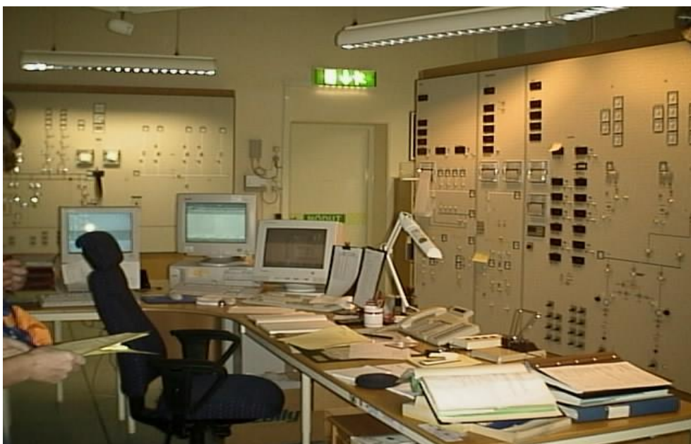
Figure 9.1 The control room in Älvkarleby hydro power plant
