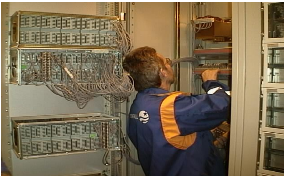
Figure 9.2 A typical work environment for a service technician in a hydro power plant
